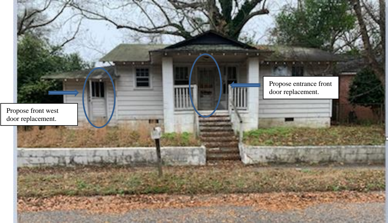
Attachment F: Two front doors (entrance door and door to the west)
