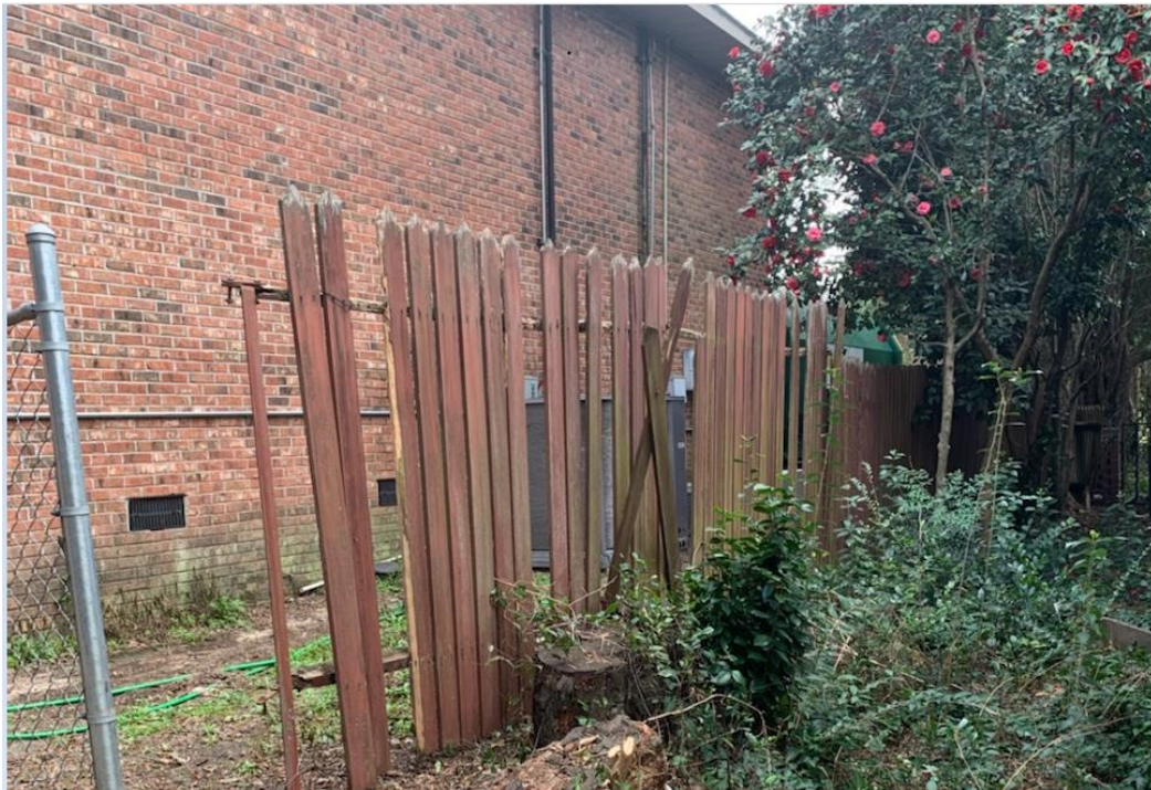
Wooden fence to be replaced
