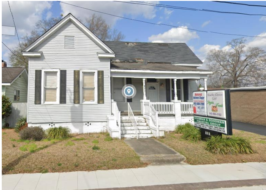
Street view photo showing the damaged shingle roof.
