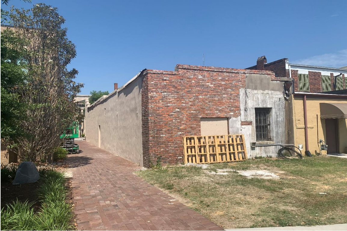
Current Rear Façade of 124 North Dargan Street and Alley Way between 114 North Dargan Street
