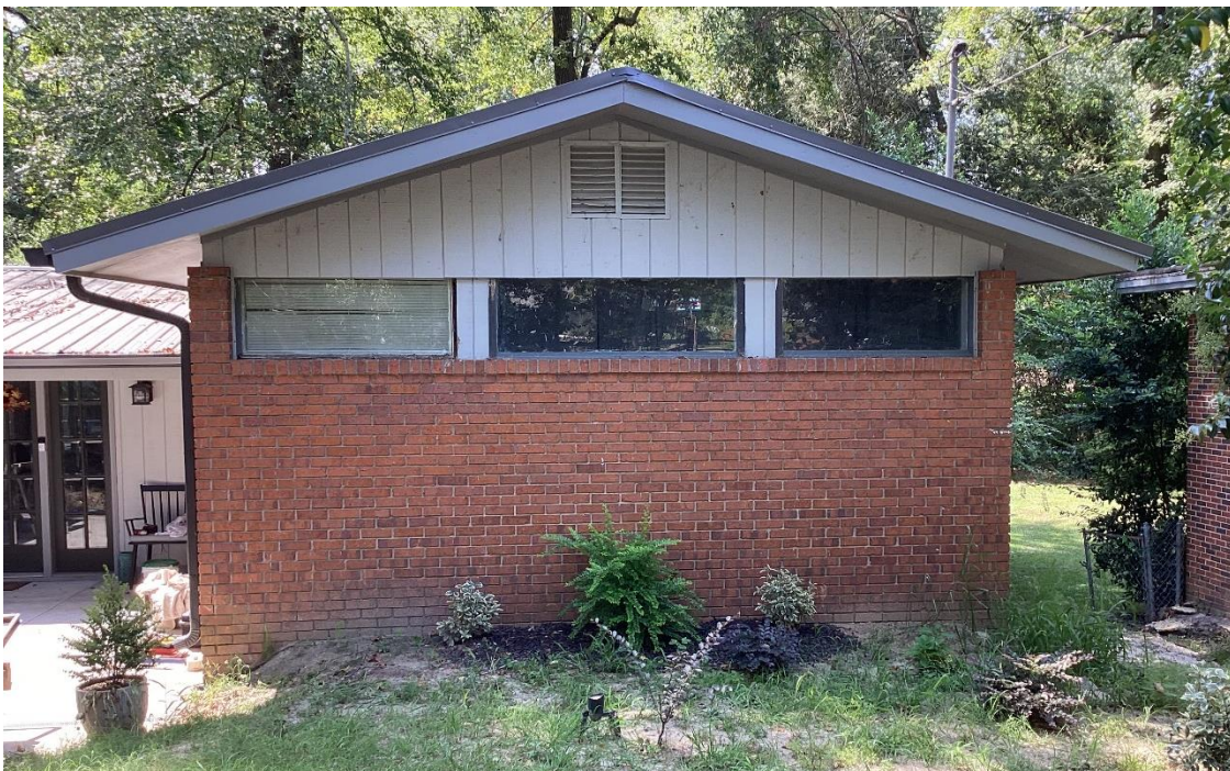
The right side of the house with the windows to be removed. The siding is to be expanded to infill the wall instead of the windows.
