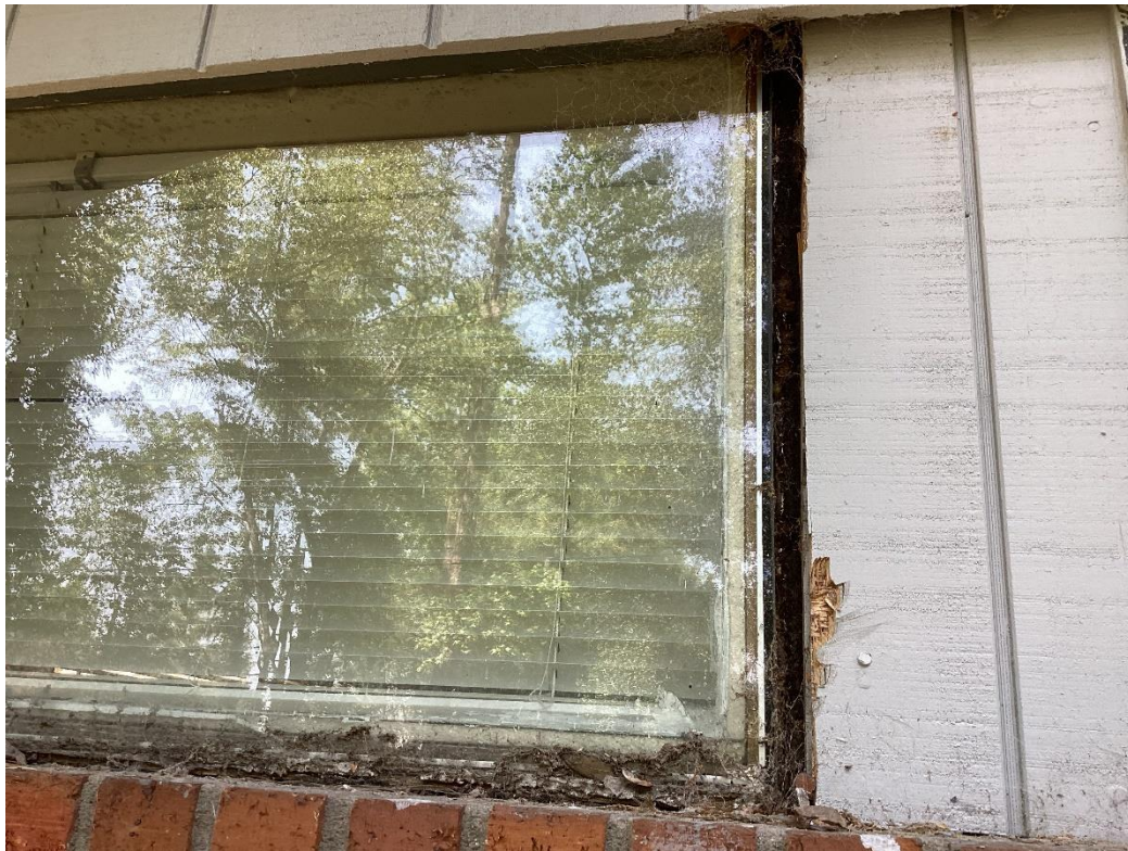
A closeup showing the damage around the windows and the existing siding.
