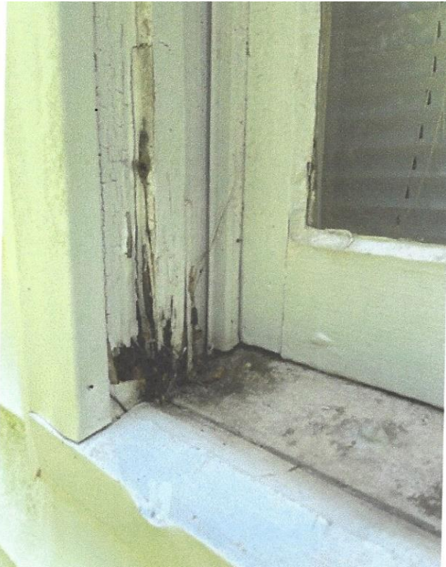
Attachment E: Site photos of the rotten window casing
