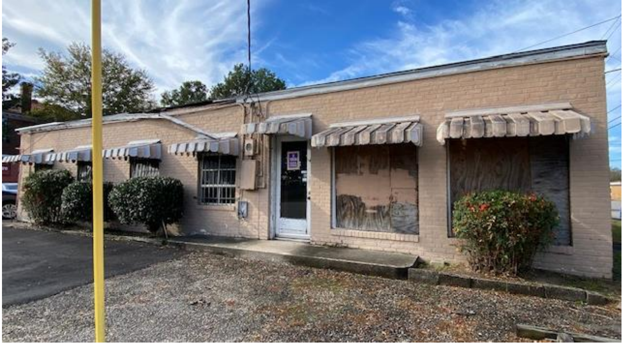
Side facing South McQueen Street. The two picture windows are missing.
