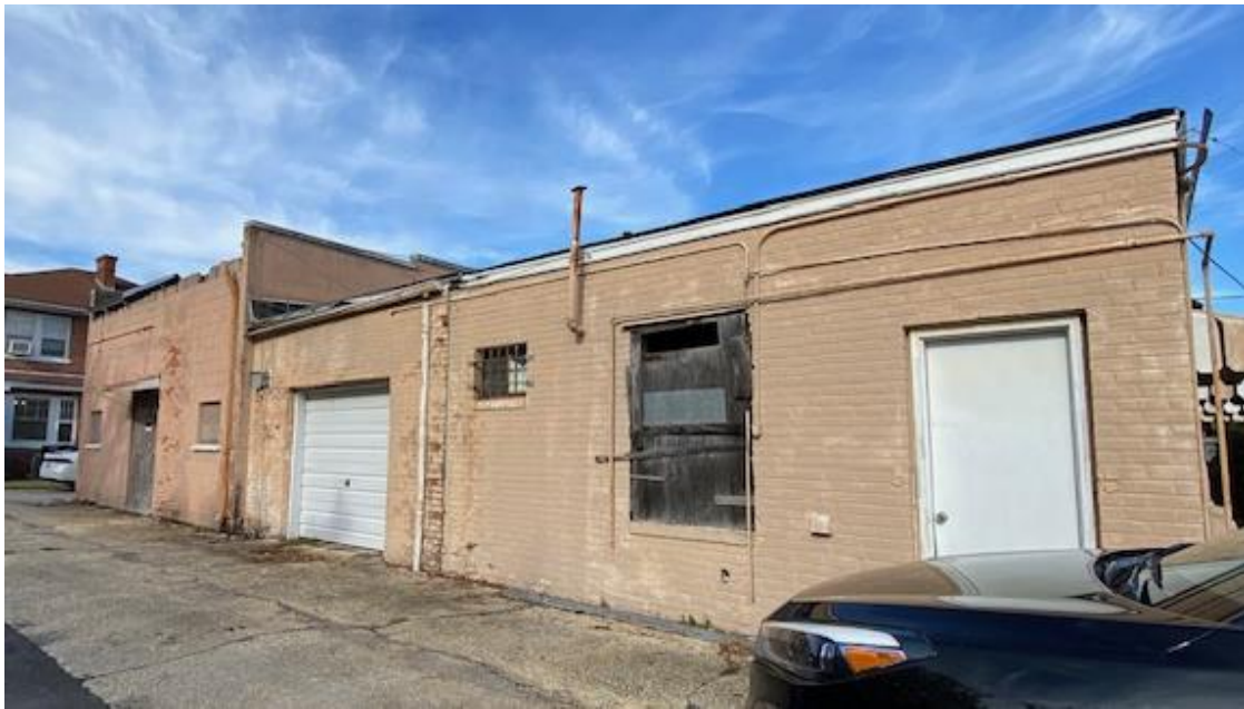
Rear of building. The brick portion will be renovated; the stucco portion on the left is to be demolished.
