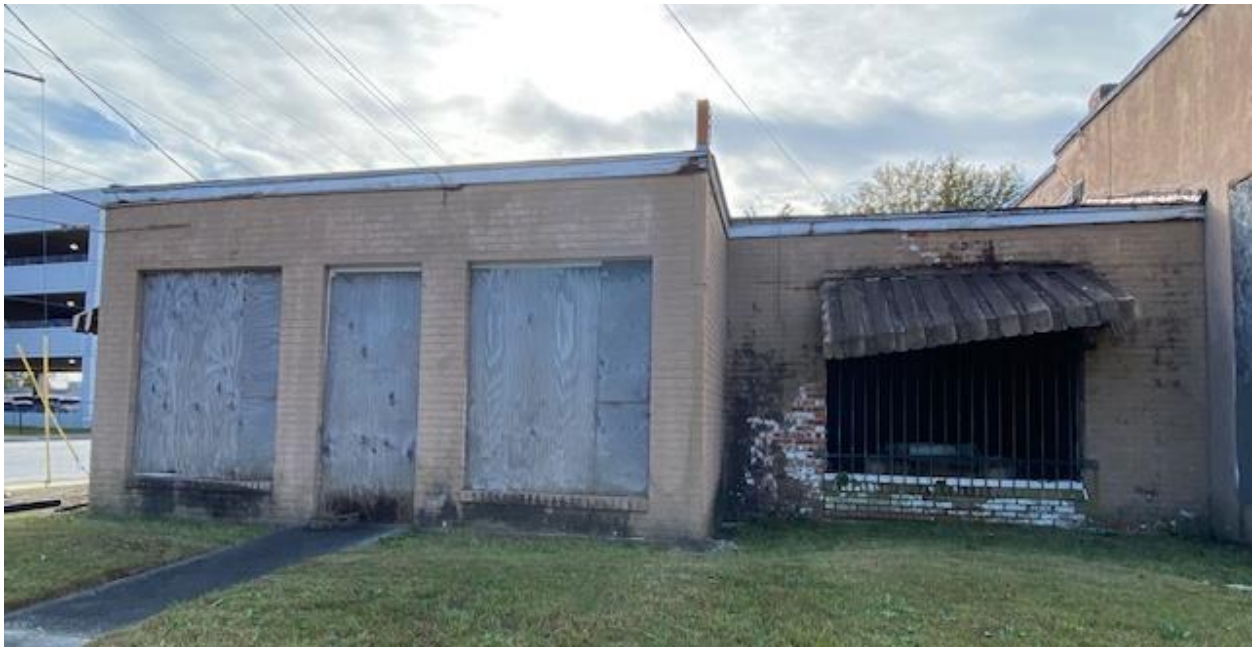
Front facing West Cheves Street. The windows and door are all missing.
